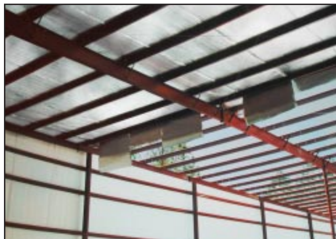
Photo #3: Reflective insulations are installed in metal buildings without a support structure such as poultry netting. These products are self-supporting and should be tested for their flame spread performance without additional support.
